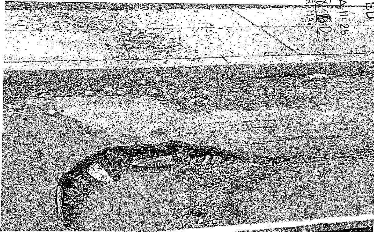
Pothole on Twelfth Street
